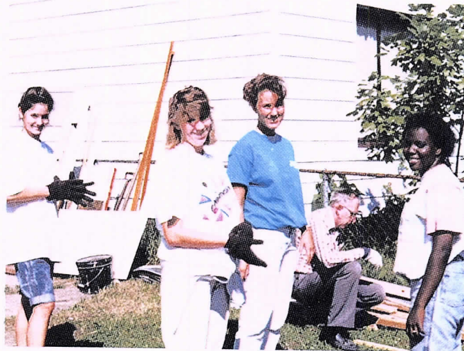
Students from DePauw University do whatever is needed, from building a new fence to digging trenches for sewer lines or finishing indoor painting. And they smile as they work.
