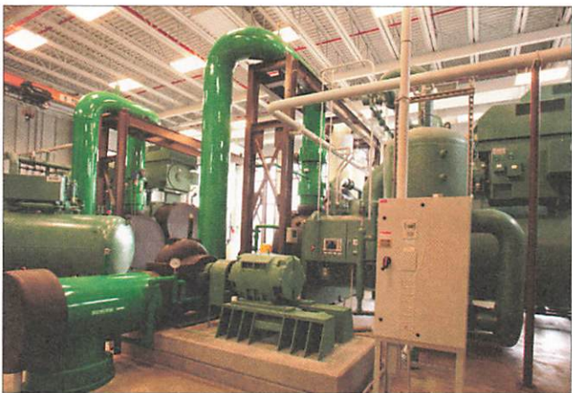
Ball State University geothermal heat pumps
